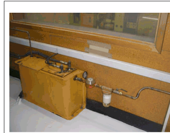
Running tank for Unit 3 (Units 1 & 2 are the same) These will be connected to the new day tank
