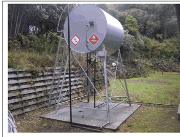
Existing day tank Showing pipework and sensors
