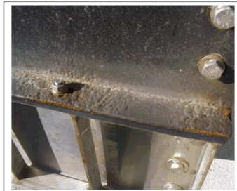
Rust on Unit 4 cooling tower
