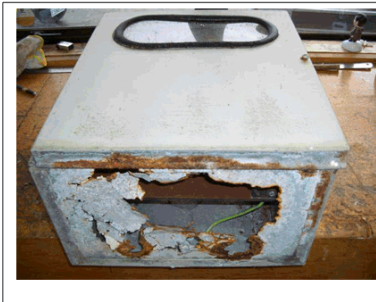
The meter box from 3 Willet Street
