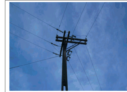
Pole 808063 drop out fuses where a connection failed on 23 September
