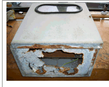
The meter box from 3 Willet Street
