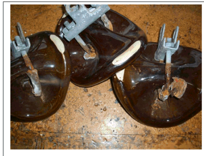
High Voltage "kidney strain" insulators in poor condition
