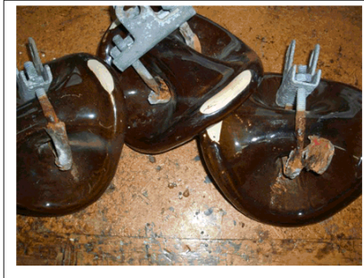
High voltage "strain" insulators from Pole 808064 showing corrosion of metal fittings
